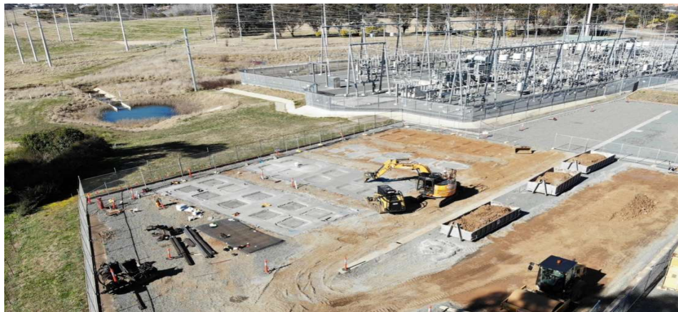
*Works on the foundations for the Battery Energy Storage System at Queanbeyan Substation
