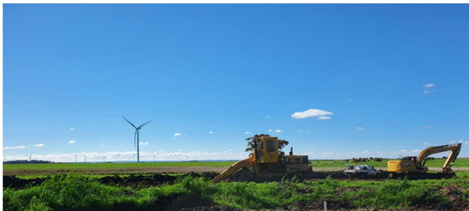
*Berrybank Stage-2 Wind Farm Cable Trenching with Berrybank Stage-1 Wind Farm in the background
